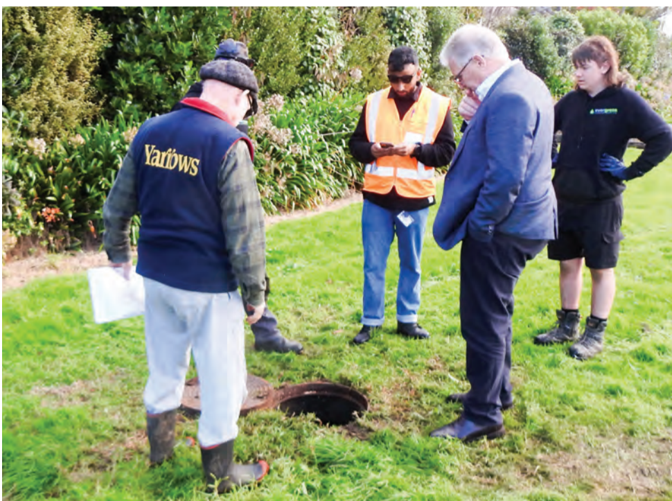
South Taranaki District mayor Phil Nixon looks into the offending manhole.
